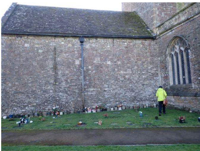
Fig. 18. Windowless north chancel wall showing a variety of stone, including squared blocks of ?Dundry Stone. Stone tile roof also well displayed.
