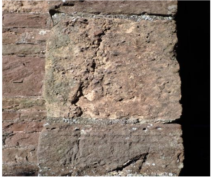
Fig. 17. buttress in south nave composed of blocks of Tintern Stone and Dolomitic Conglomerate.
