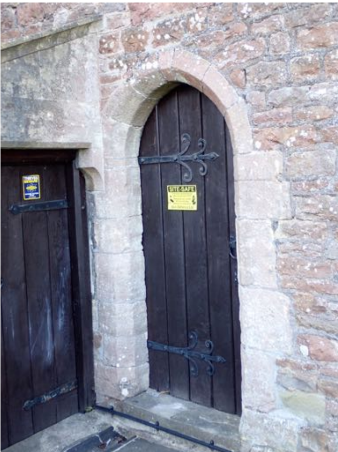
Fig. 22. Dundry Stone doorway in south wall of chancel with Sudbrook Stone in 1 and 2 o'clock positions.
