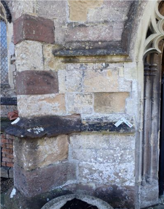
Fig. 14. Close up of stone in porch buttress. Red = Tintern Sandstone, yellow = Dolomitic Conglomerate, Cream = Dundry Stone. Doorway Bath Stone.
