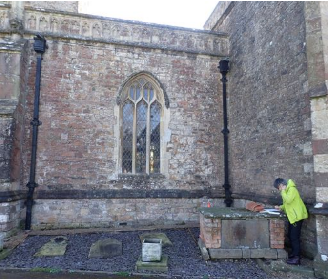
Fig. 15 Nave, fabric dominantly Carboniferous Limestone, locally reddened by a coating of algae, string course of Tintern Sandstone and battlements of ? Dundry Stone.
