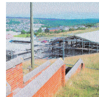
Above: a brand new office block and conservation area under construction at Big Pit
