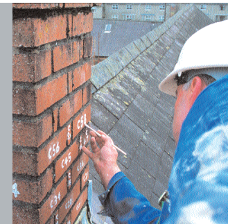
Above: to enable later re-erection, a chimney at the Museum of the Welsh Woollen Industry is carefully recorded before being taken down
